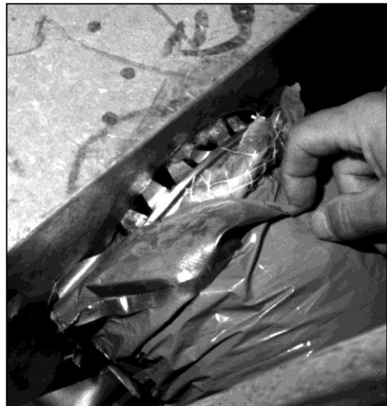
Supply Leak at Take-Off Connection
