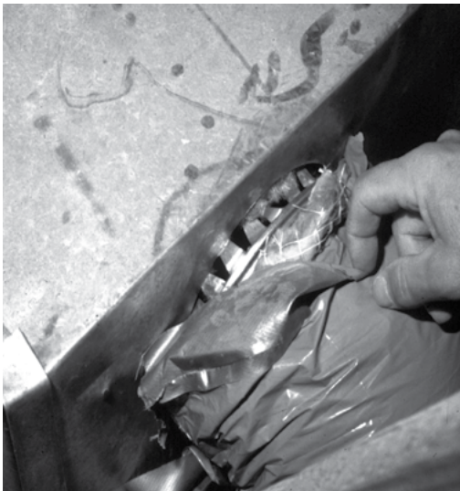
Return Leak Through Wall Cavity
