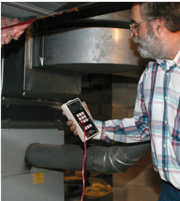
Figure 5. A digital manometer is used to measure the oil-fired furnace's draft, or ability to vent combustion gases.
